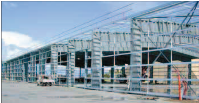
An example of the ILB system at a Townsville construction site.
